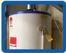
Gas water heater
